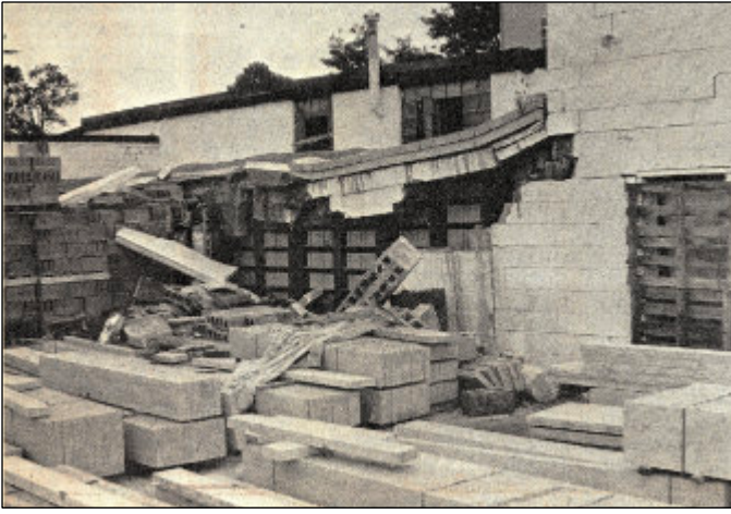
A photo from the Canadian Statesman , August 1, 1979 shows the damage to Newcastle Cement Block following a propane gas explosion which badly injured owner Bert De Bruin.
